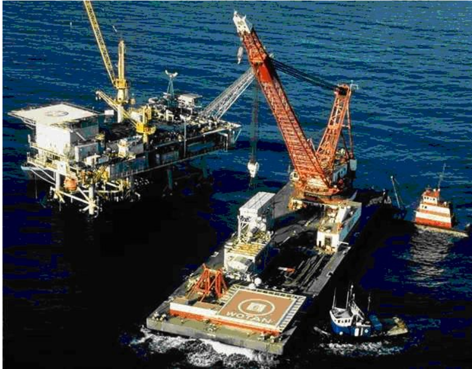
Figure 22 - Manson Construction 600 ton Derrick Barge WOTAN operating offshore (courtesy of Manson Construction)
